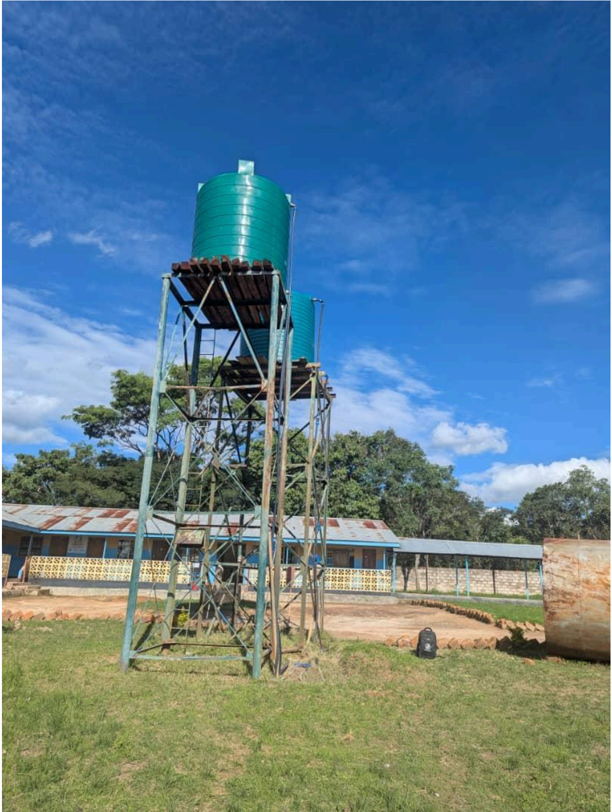
WATER TANK ON THE STAND WITH WATER
